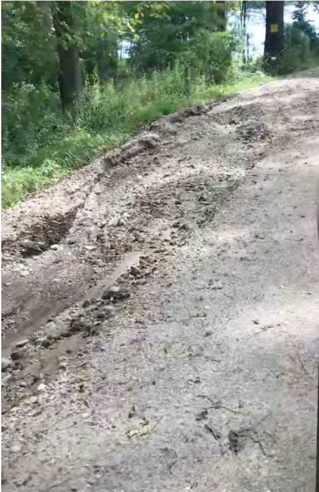
PHOTO 2 - Roadway shoulder washout
