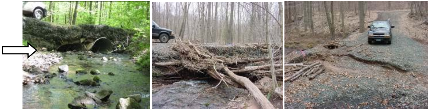
Figure1. Collapsing culverts in Brooksvale Stream (left photo), clogged by woody debris (middle photo), causing the road to wash out (right photo). Photos by Gerard Milne.
