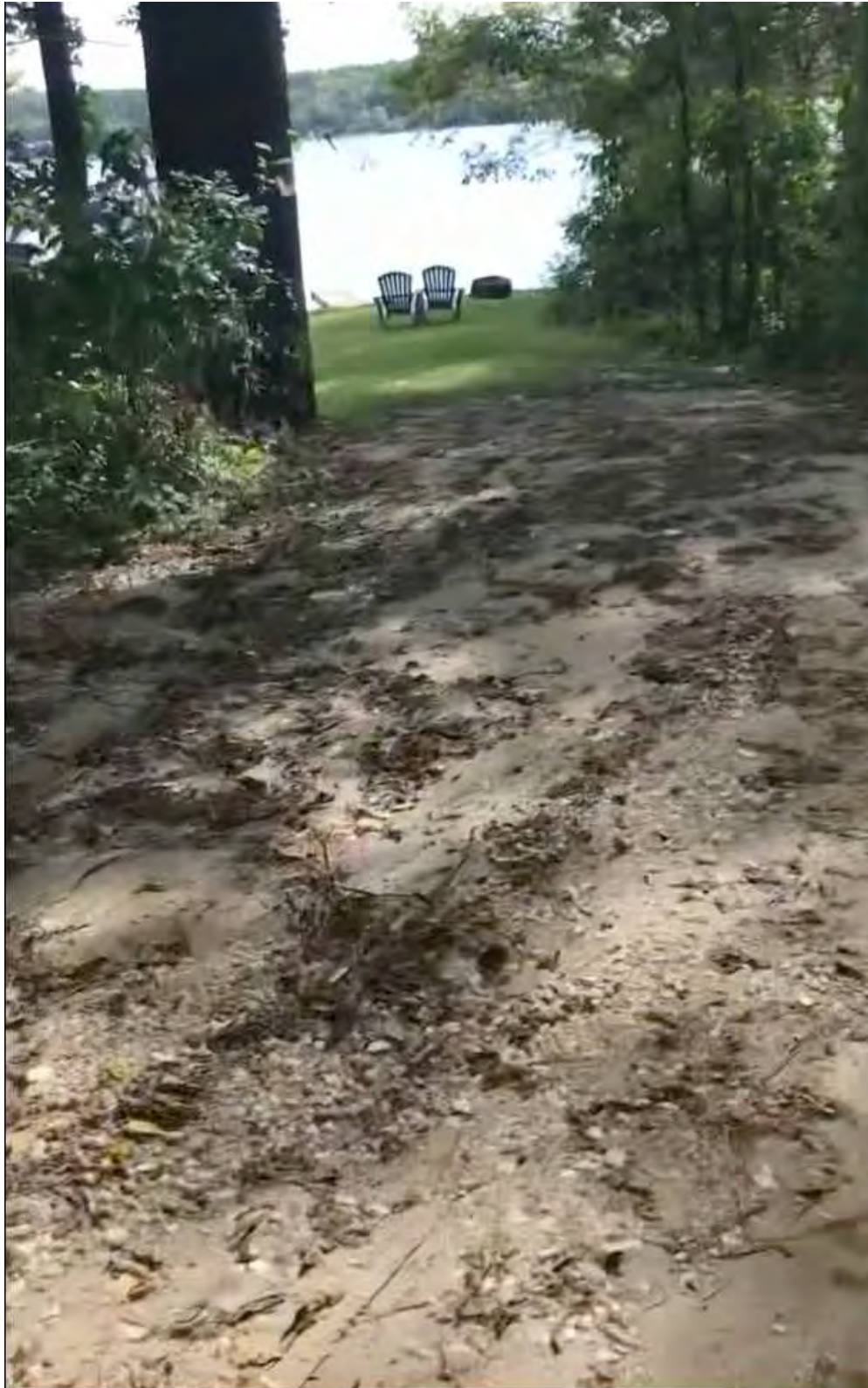
PHOTO 3 - Roadway washout onto private property
