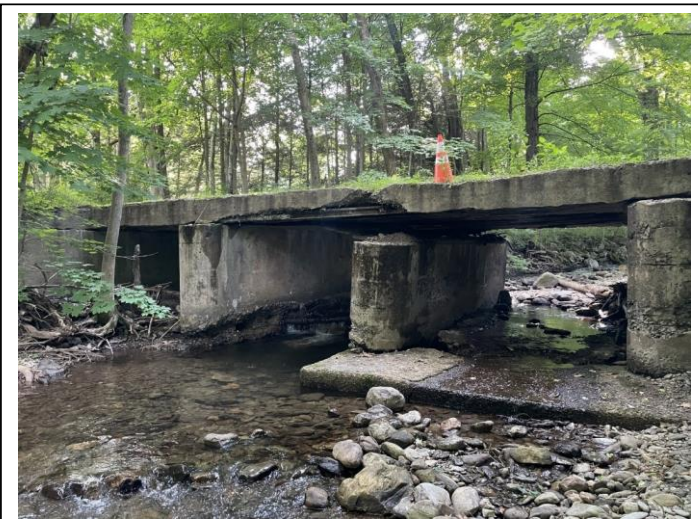
Deteriorating Rail Trail bridge (note safety cone) over Wachocastinook Brook. - Rehabilitation of this bridge could provide multimodal access to the Pope Property. Photo: Tracy Brown
